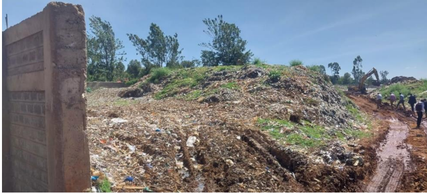
Figure 2: Photo showing huge heaps of garbage and a bull dozer doing some works on the dumpsite
